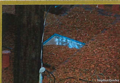
Photo 1. Accumulation of vegetative debris on top of a glass-type skylight on a low-slope roof.
